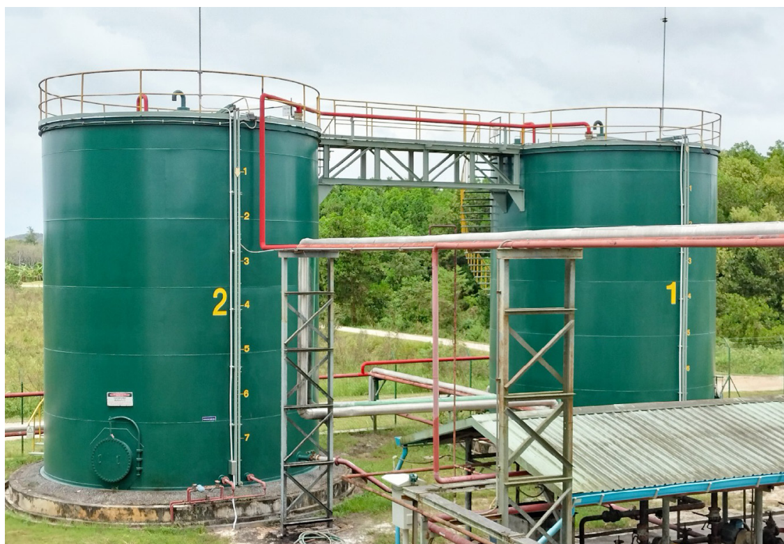
Pabon Production Tanks.
