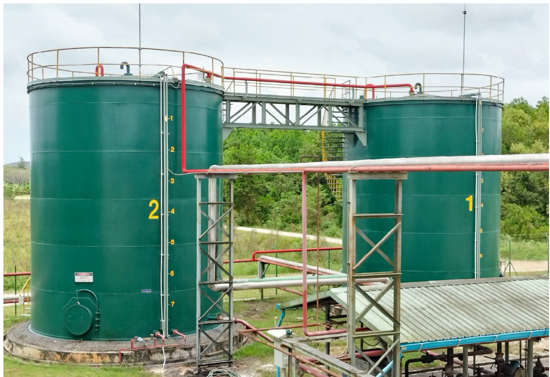
Pabon Production Tanks.
