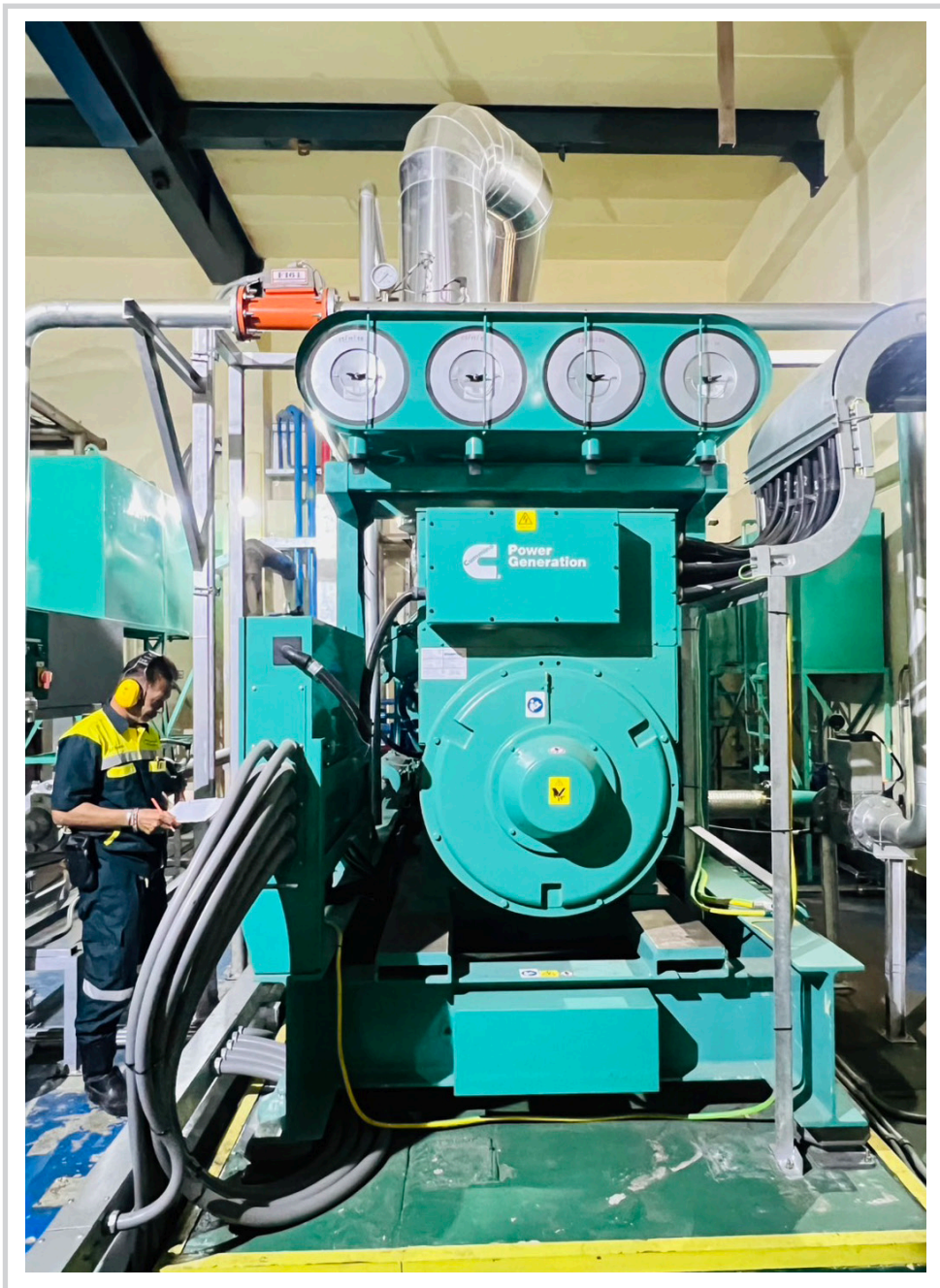
Topi Replacement Gas Engine
