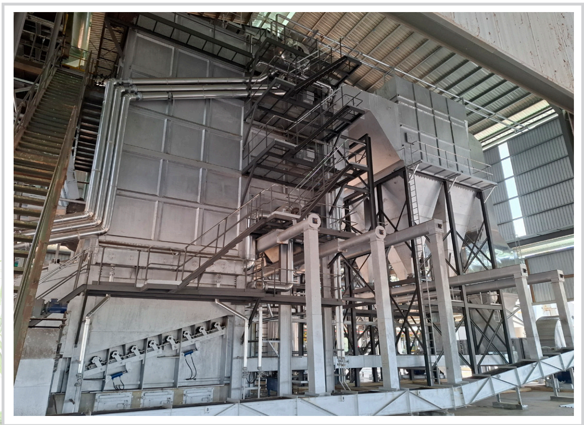
Cha Uat Boiler Station
